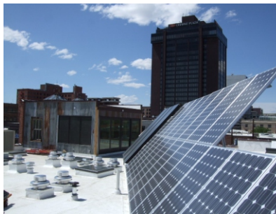
ROOFTOP PHOTOVOLTAIC DISPLAY
